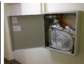
Image 2 Fire hose system cabinet
