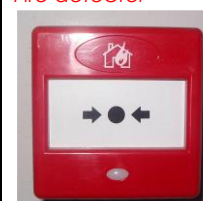
Image 5 Fire alarm button
