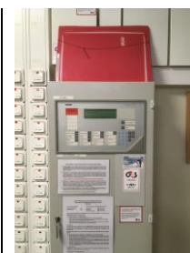
Image 3 ATS central unit
